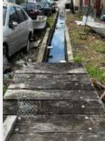
Figure 98: Surface water drainage from Harmony Hall & Bamboo Road (Urban environment) discharging into the swamp as part of flood mitigation
