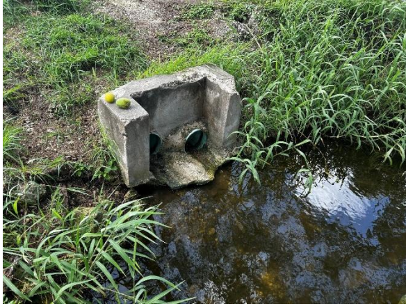
Figure 6: Surface water drainage from Harmony Hall & Bamboo Road (Urban environment) discharging into the swamp as part of flood mitigation
